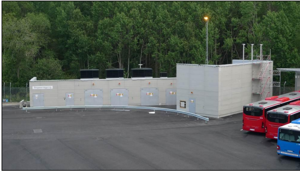
Figure 12. Compressors and LNG back-up storage at Gubbängen depot.
