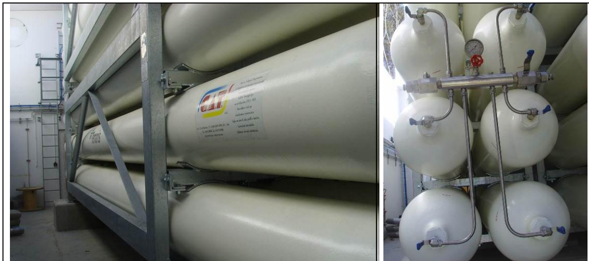
Figure 5. Stationary gas storage with horizontal gas bottles at Gubbängen depot.
