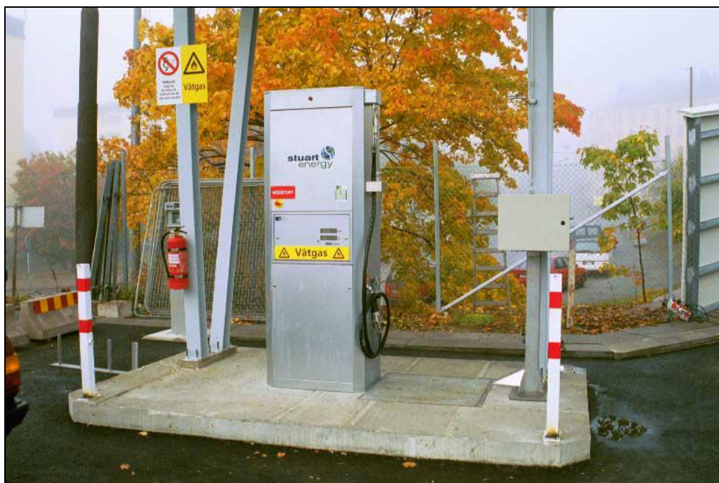
Figure 7. Hydrogen refuelling station in Stockholm.
